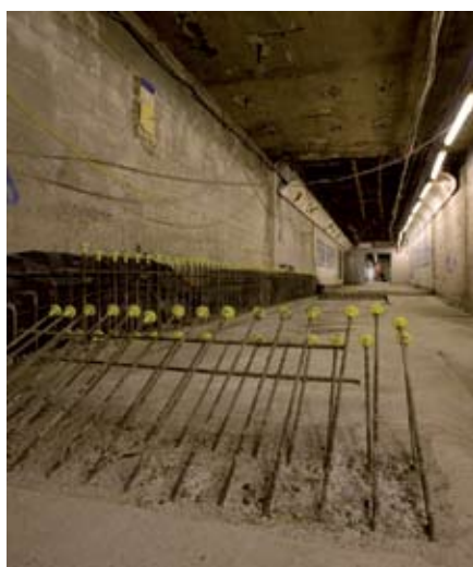
The disused eastern subway will be restored and re-opened in time for the Games to reduce congestion and make it easier to change between services
