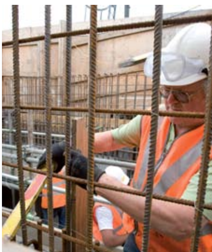
Workers install steel reinforcements for new lifts and stairs to go from platform 6/8 into the disused eastern subway (due to be reopened by 2010)
