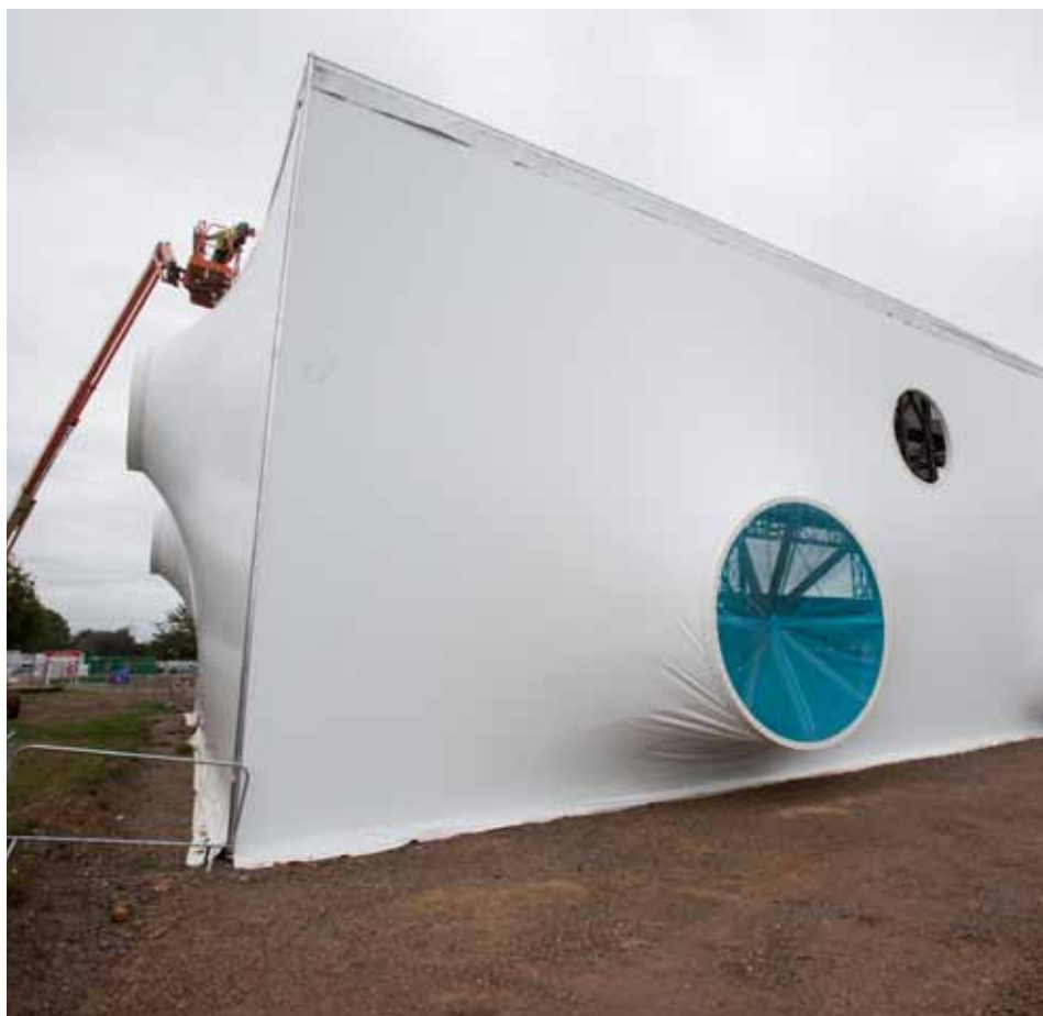
Construction is well underway on the temporary facilities, with cladding now being installed on the indoor ranges
