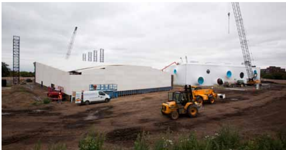
Construction is progressing well on the London 2012 Shooting and Paralympic Archery venue
